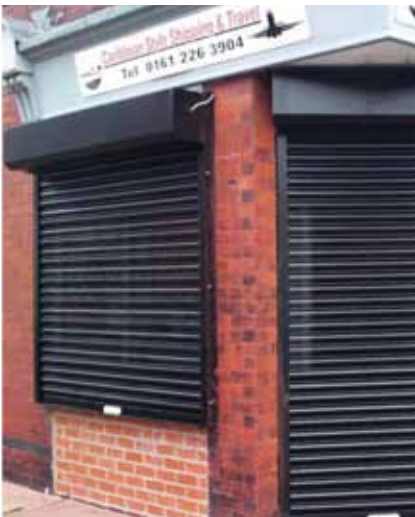
Image of bad grill shutter installations
